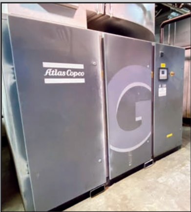
(2) ATLAS COPCO 200 HP ROTARY SCREW AIR COMPRESSORS
