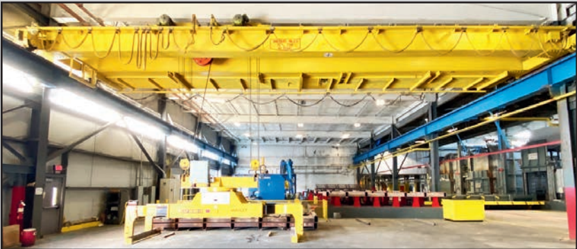
SAMPLE BRIDGE CRANE
